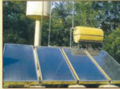
Solar Water Heater
