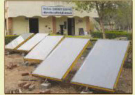
Solar Flat Plate Collectors
